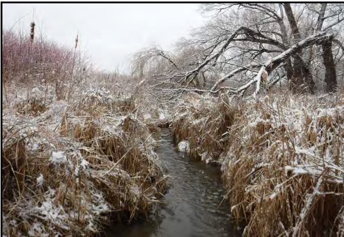
PHOTOGRAPH NO.: 16 - Culvert 9 FROM: Upstream end of culvert LOOKING: Upstream at channel COMMENT:
