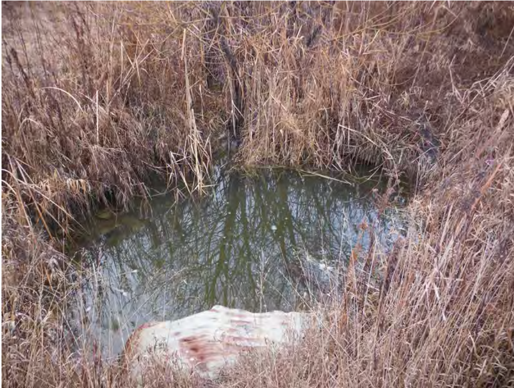
PHOTOGRAPH NO.: 13 - Culvert 7 FROM: Huntington Road LOOKING: Upstream of Culvert COMMENT: Rainbow Creek
