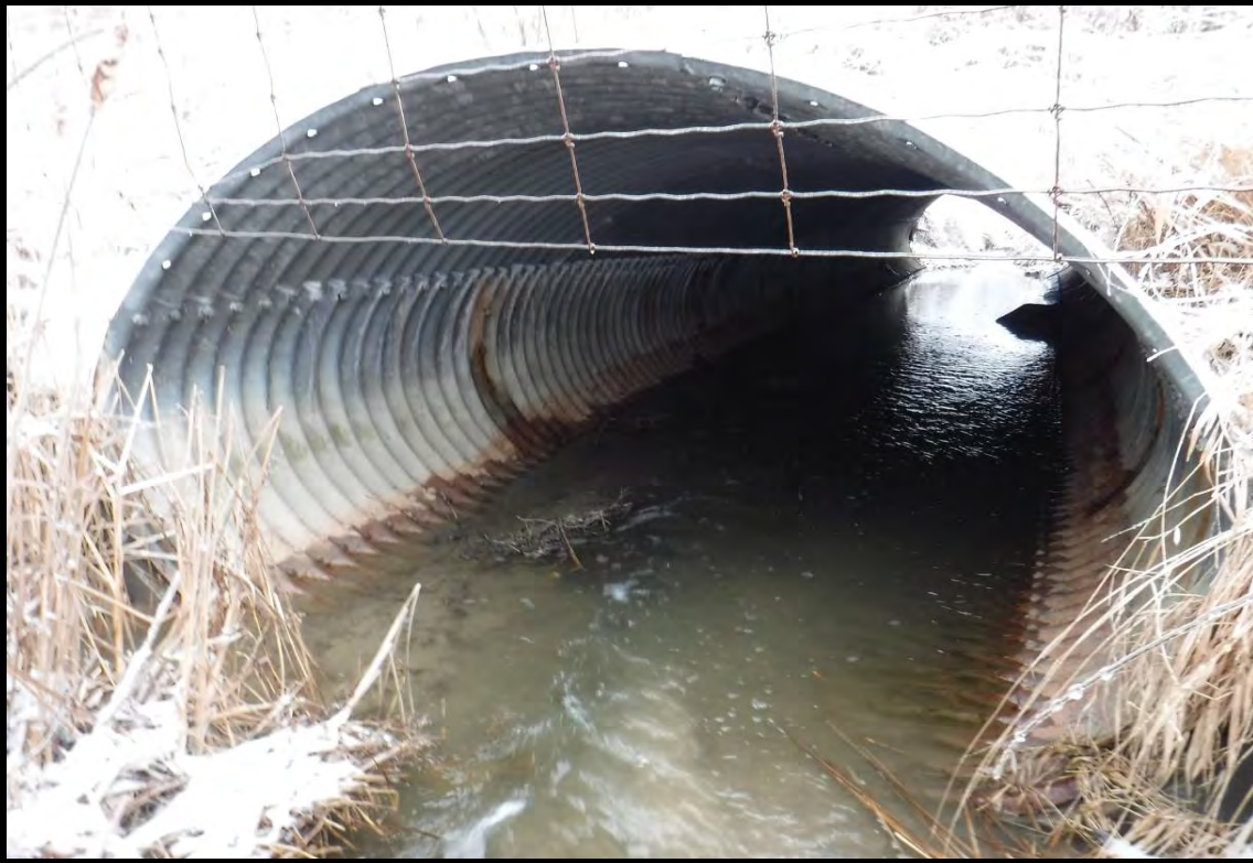
PHOTOGRAPH NO.: 17 - Culvert 9 FROM: Upstream of culvert at road LOOKING: Downstream at culvert COMMENT:
