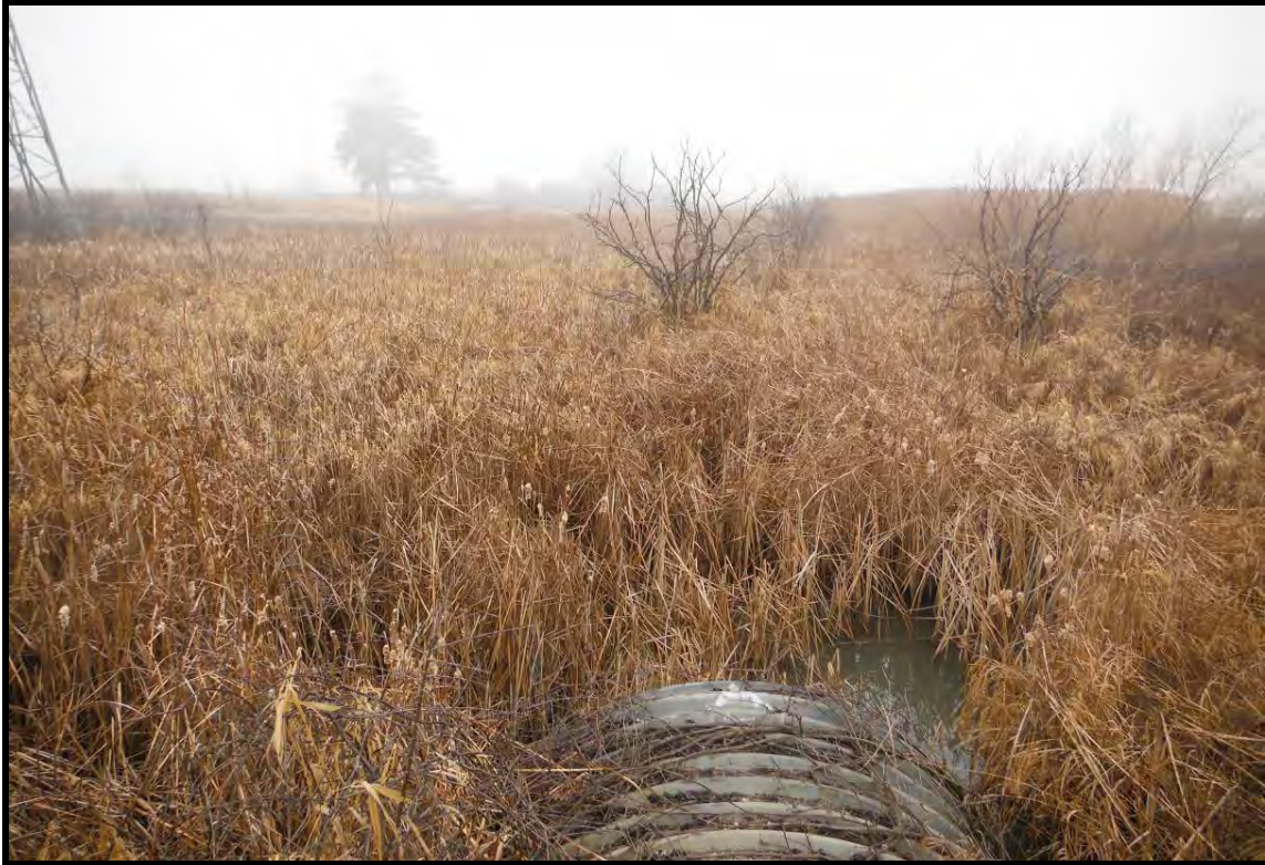
PHOTOGRAPH NO.: 9 - Culvert 6 FROM: From upstream end of culvert LOOKING: Upstream COMMENT:
