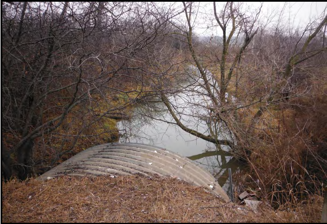
PHOTOGRAPH NO.: 7 - Culvert 5 FROM: Downstream end of culvert LOOKING: Downstream at channel bed COMMENT: Active grazing lands
