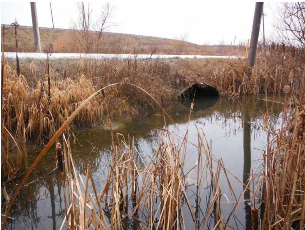
PHOTOGRAPH NO.: 14 - Culvert 7 FROM: Huntington Road LOOKING: Downstream of Culvert COMMENT: Rainbow Creek Tributary
