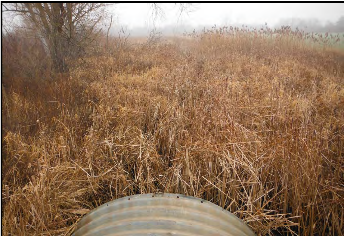
PHOTOGRAPH NO.: 10 - Culvert 6 FROM: Downstream end of culvert LOOKING: Downstream at channel COMMENT:
