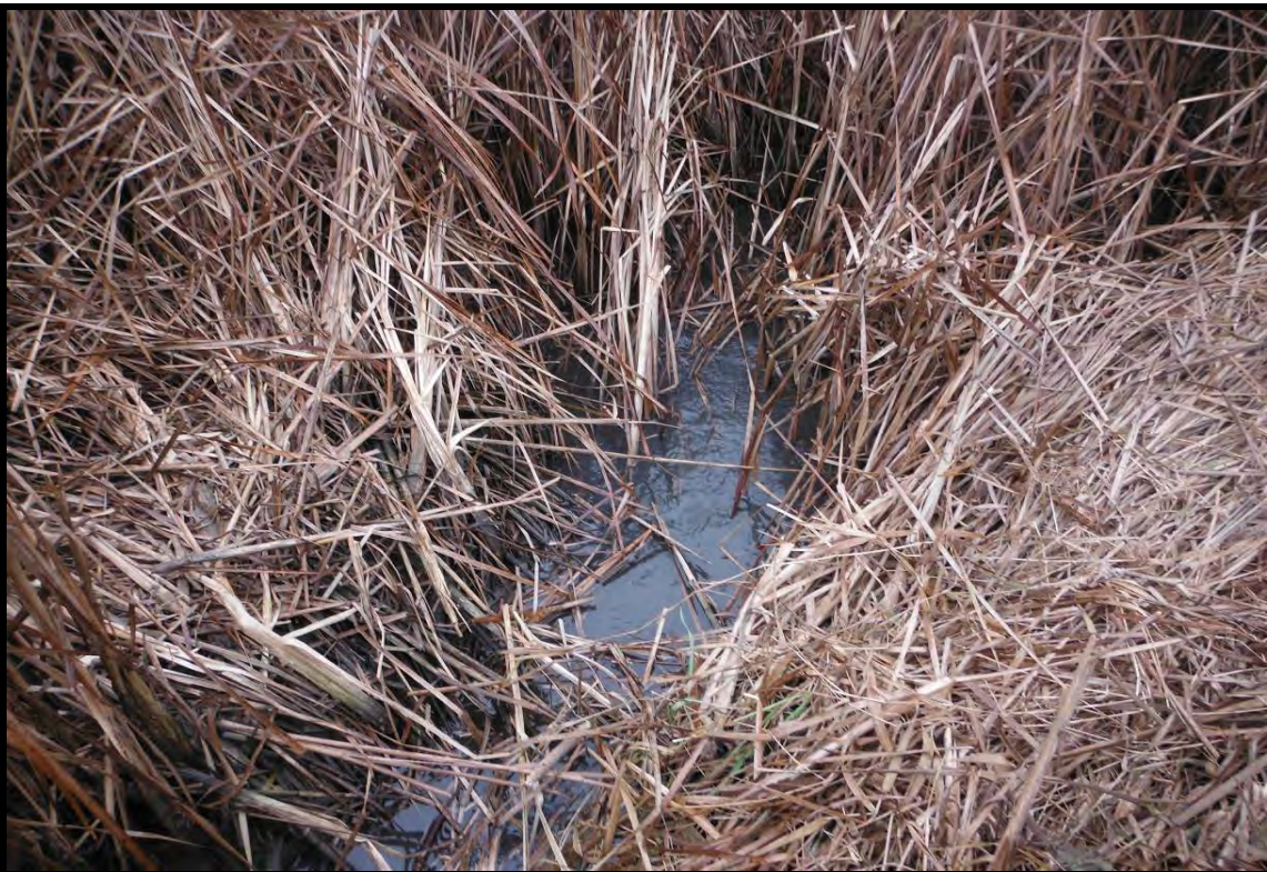
PHOTOGRAPH NO.: 12 - Culvert 6 FROM: Downstream end of survey LOOKING: Upstream at channel COMMENT: Typical shape of channel through reach
