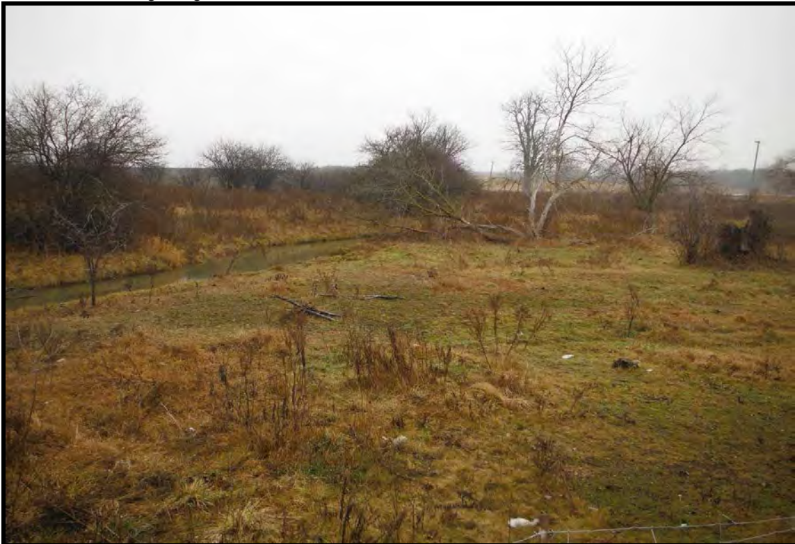
PHOTOGRAPH NO.: 8 - Culvert 5 FROM: From road LOOKING: Downstream at channel through grazing lands COMMENT: Stream flows into online pond 50m outside of picture
