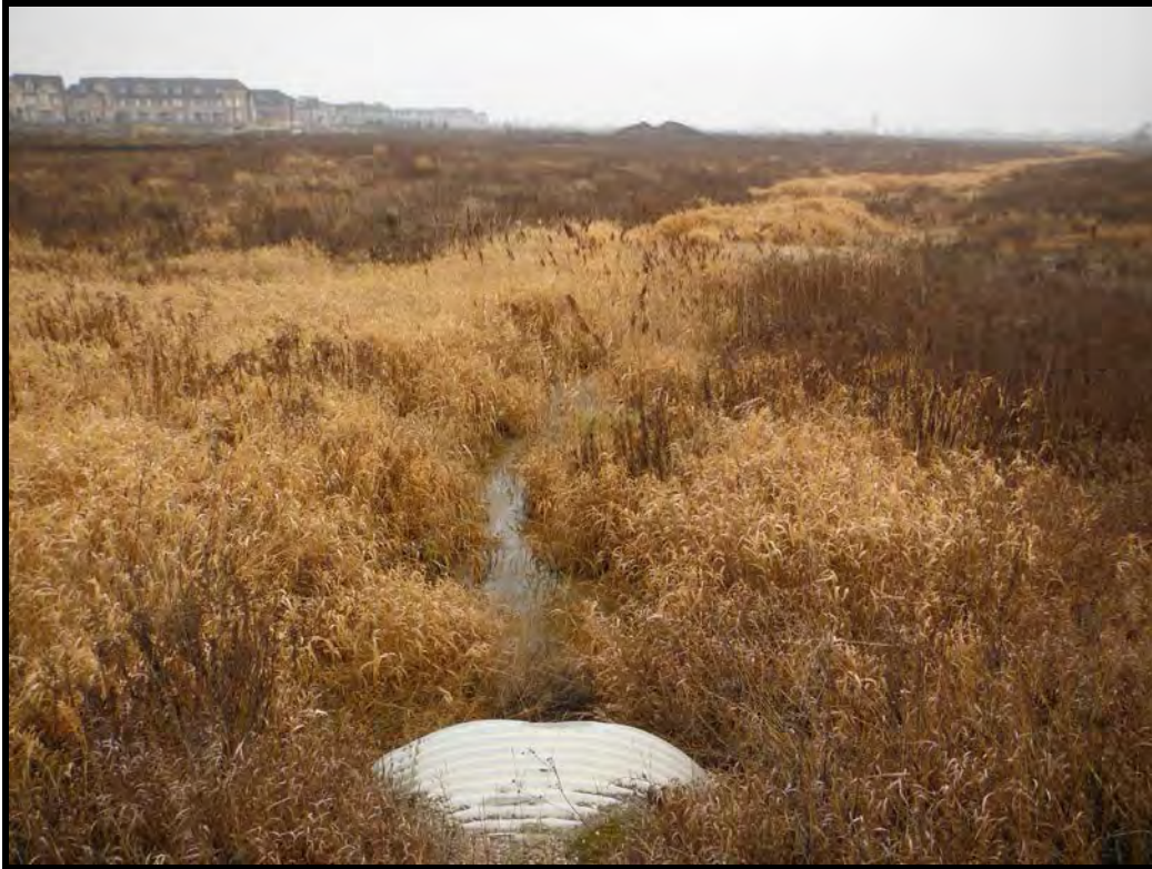
PHOTOGRAPH NO.: 1 – Culvert 4 FROM: Huntington Road LOOKING: Downstream COMMENT: East Robinson Creek
